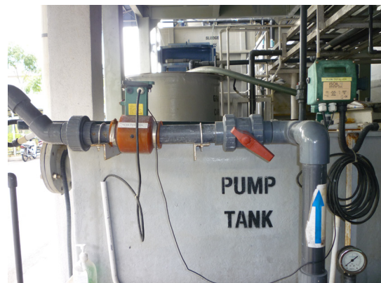
The MS5000 monitoring a small WWTP effluent line.
